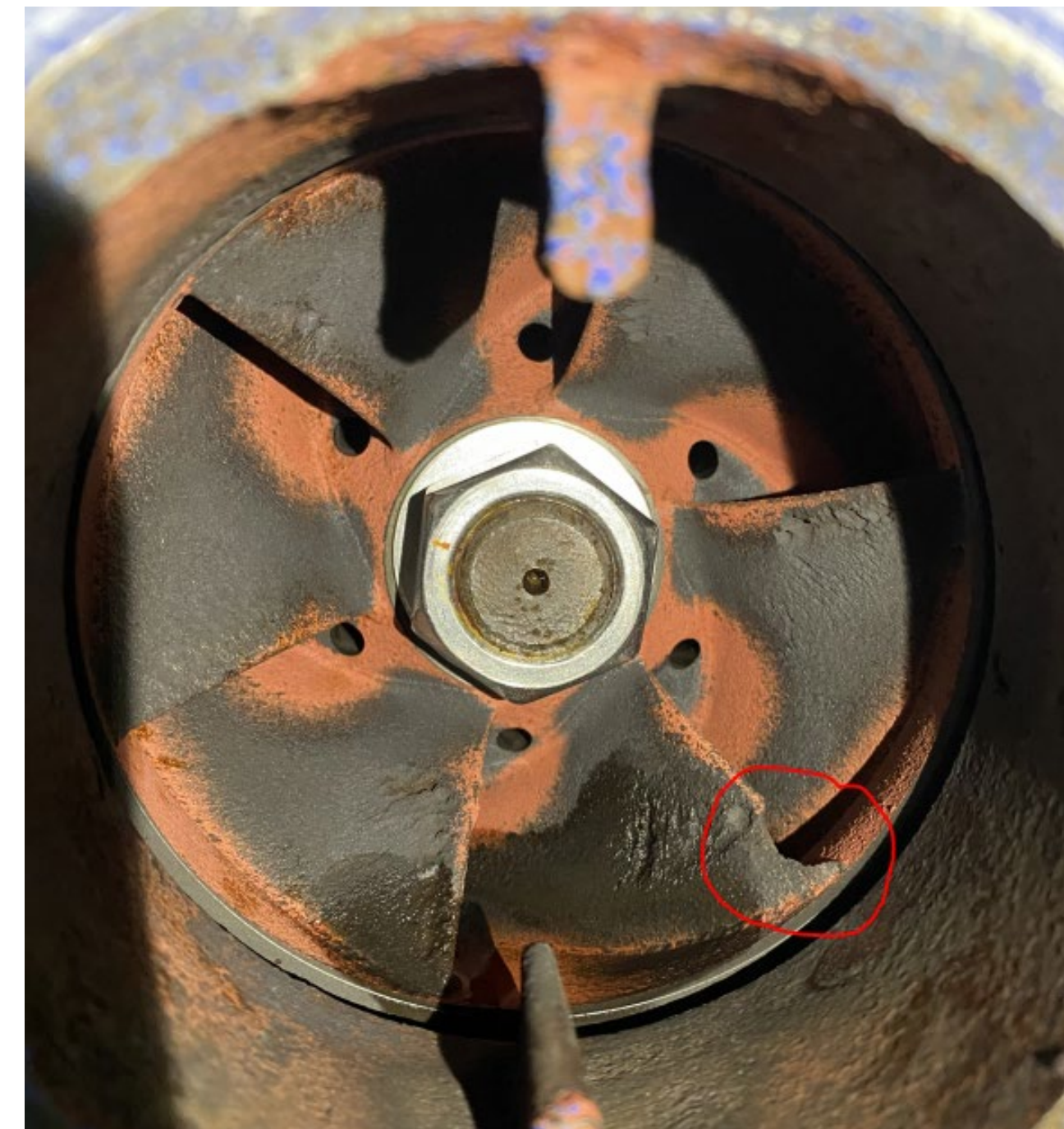
Image 3: pump with defective impeller and broken blade
